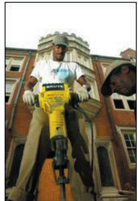
Breaking up concrete along the front foundation to make way for the new cooling system were Joelrico A. Payne, with jackhammer, and Timothy Byrd. Work began more than a year ago. (Photos by Keith Williams, The Courier-Journal)
